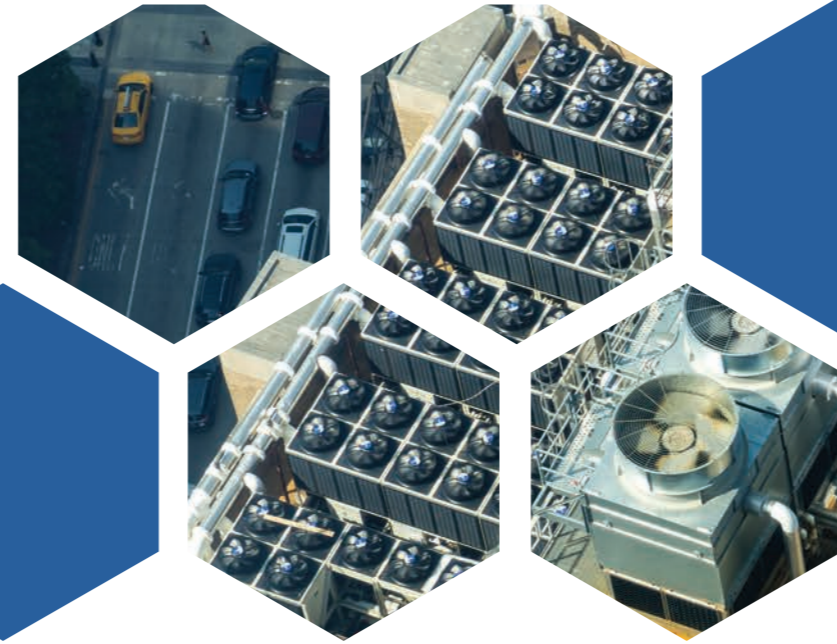
Building HVAC System
