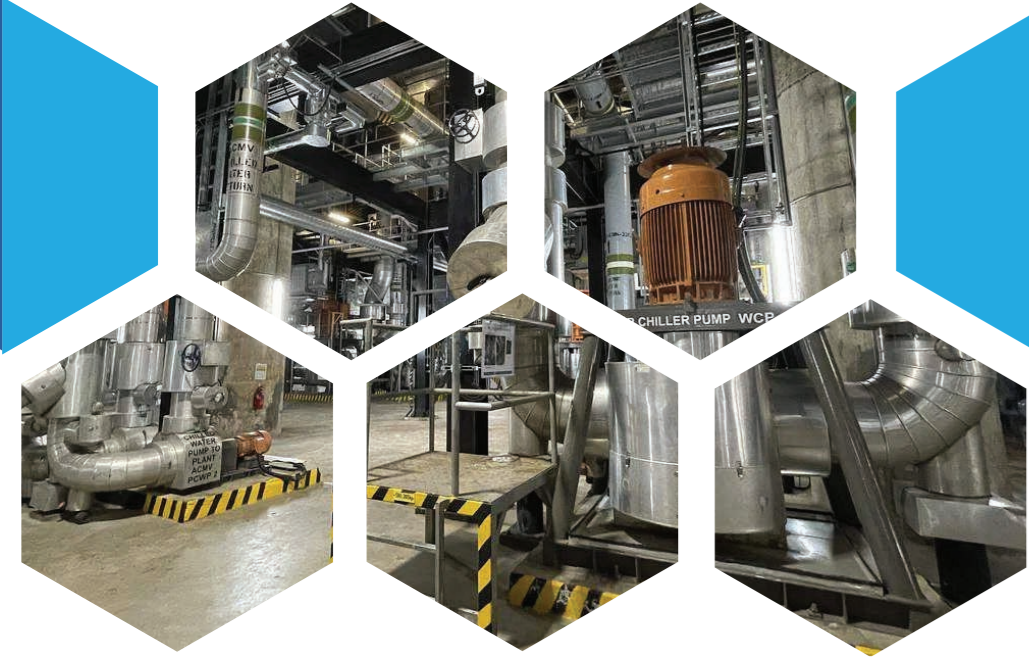
Energy Efficiency Improvement
